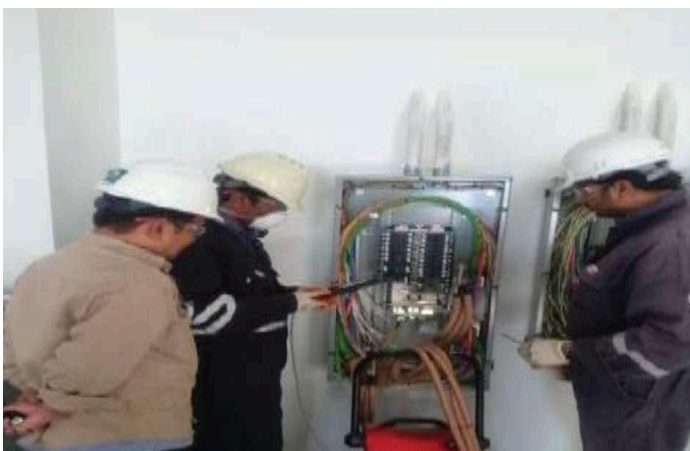
Pre-commissioning of Power Panel
