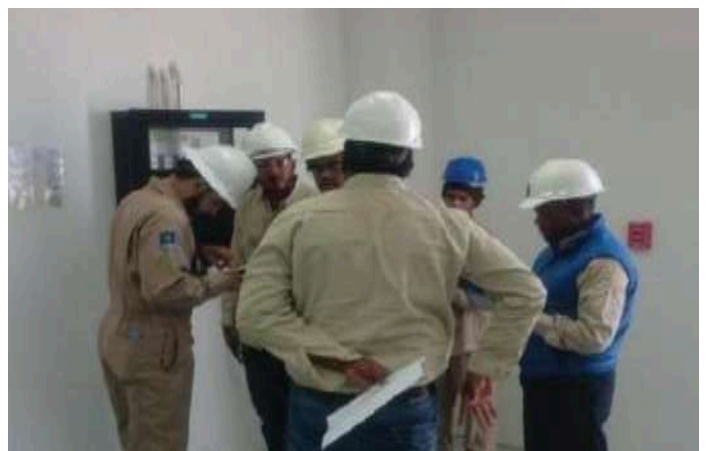
Pre-commissioning of FACP
